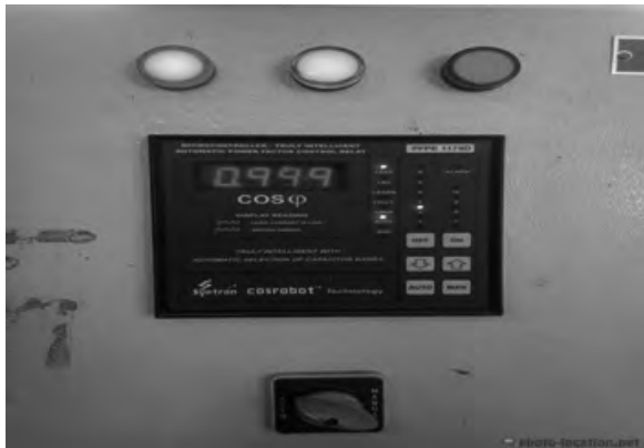
Fig. 8 APFC unit indicating unity PF
