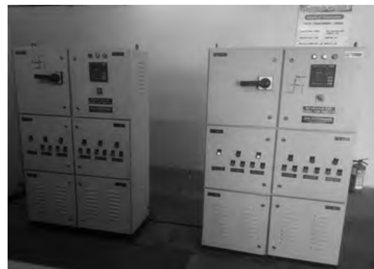
Fig. 7 30kVAR PFC unit installed with standby
